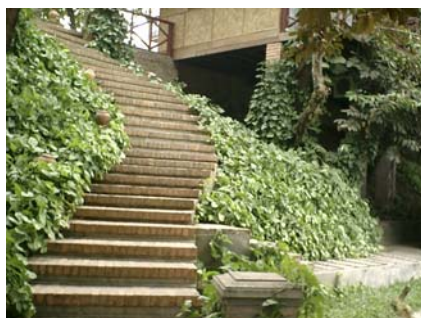
These steps are too steep and there is no handrail
