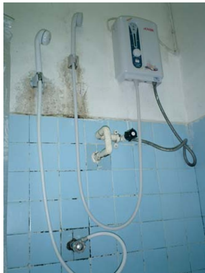
A poorly maintained shower
