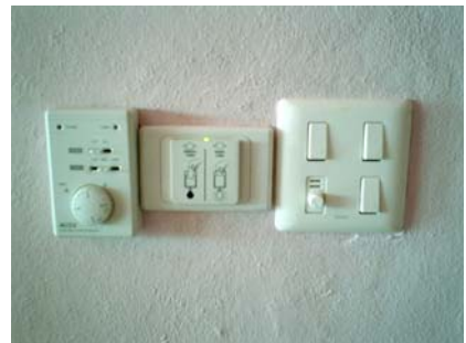
Properly installed switches
