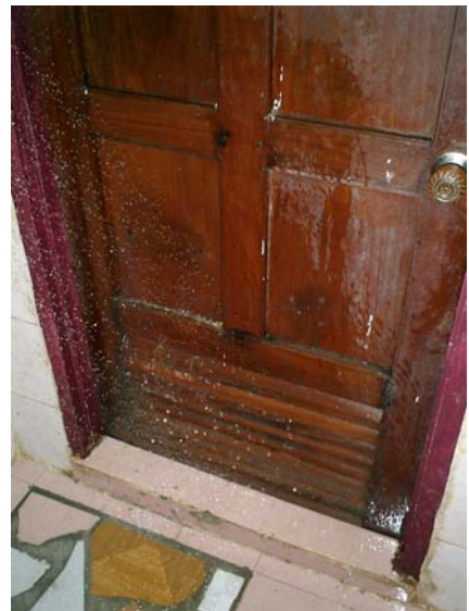
Water should not spray on the bathroom door
