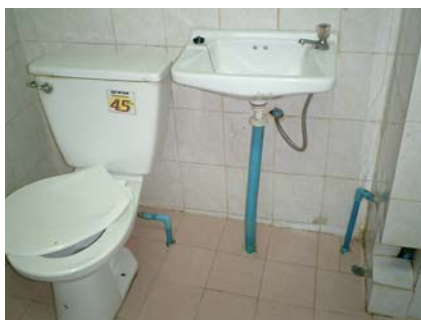
Exposed PVC pipes and broken toilet seat
