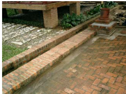
A guest can easily trip in this gutter
